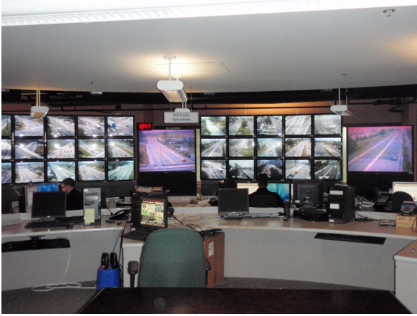
Figure 5. Operation Consoles Before Situation
