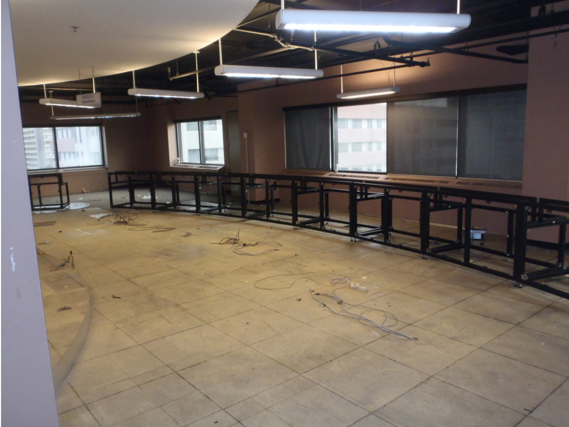
Figure 14. The Video Wall Cube Base Array
