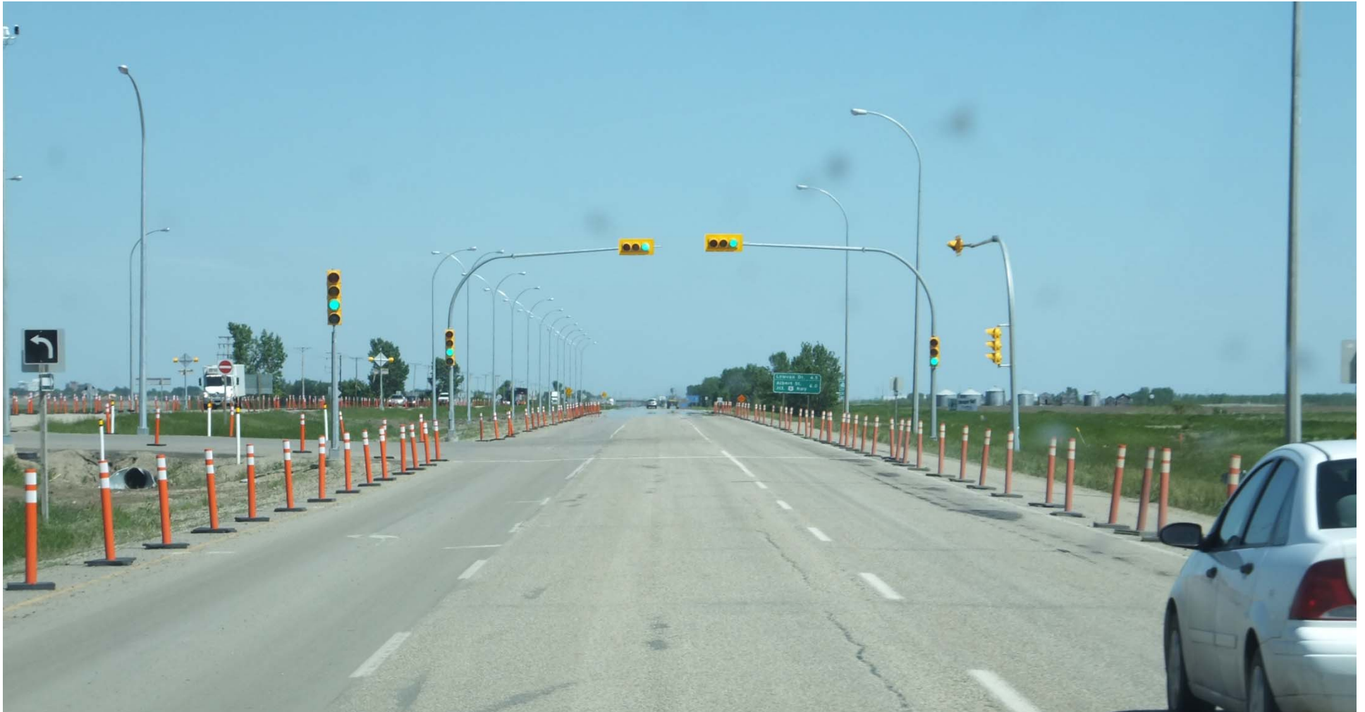
Installing Temporary Traffic Signals at a Rural Highway Intersection as an Interim Condition
