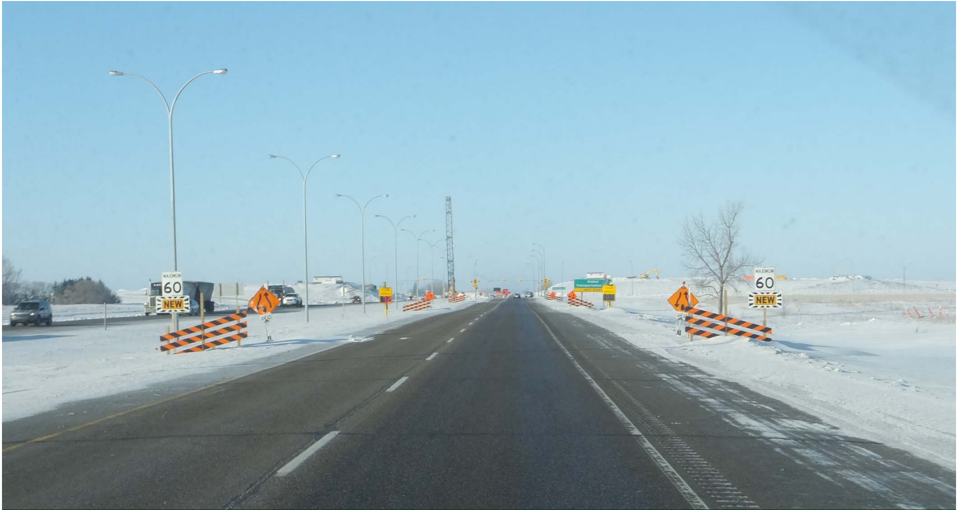
Installing Temporary Traffic Signals at a Rural Highway Intersection as an Interim Condition
