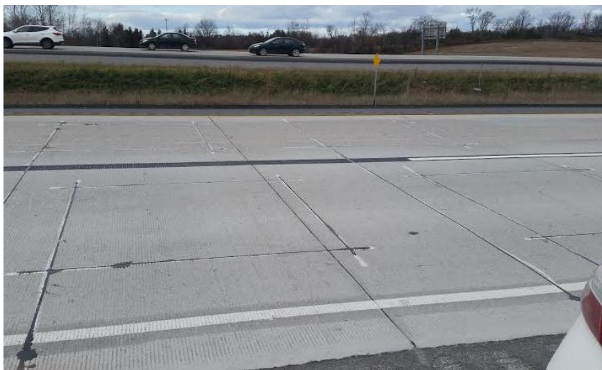
Picture 2 – Intrusive Loops on MTO's Highways
