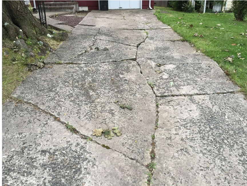
Figure 6 – Cracking due to Tree Roots [6]
