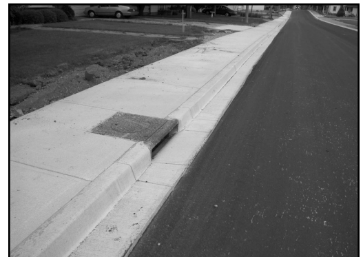
Figure 3-27. Various options exist to ensure drainage facilities do not impact the safety of cyclists.
