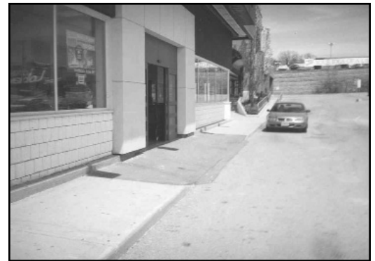
Figure 3-28. In this case, there is no separation between vehicular traffic and pedestrians at the building entrance.
